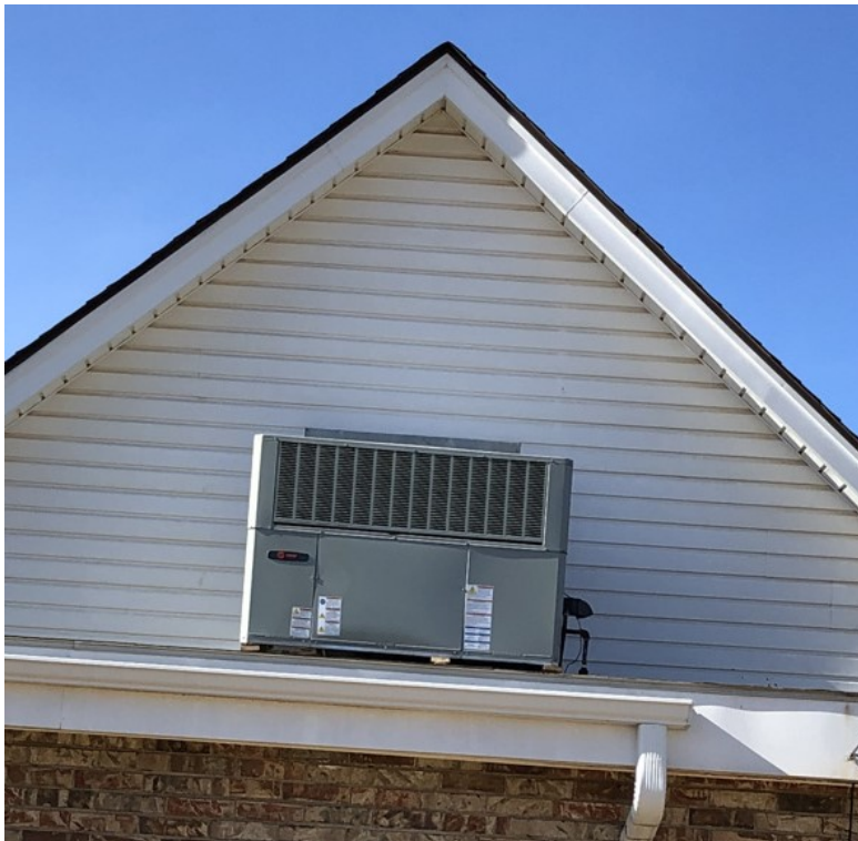
New heating/air conditioning unit for the north building
